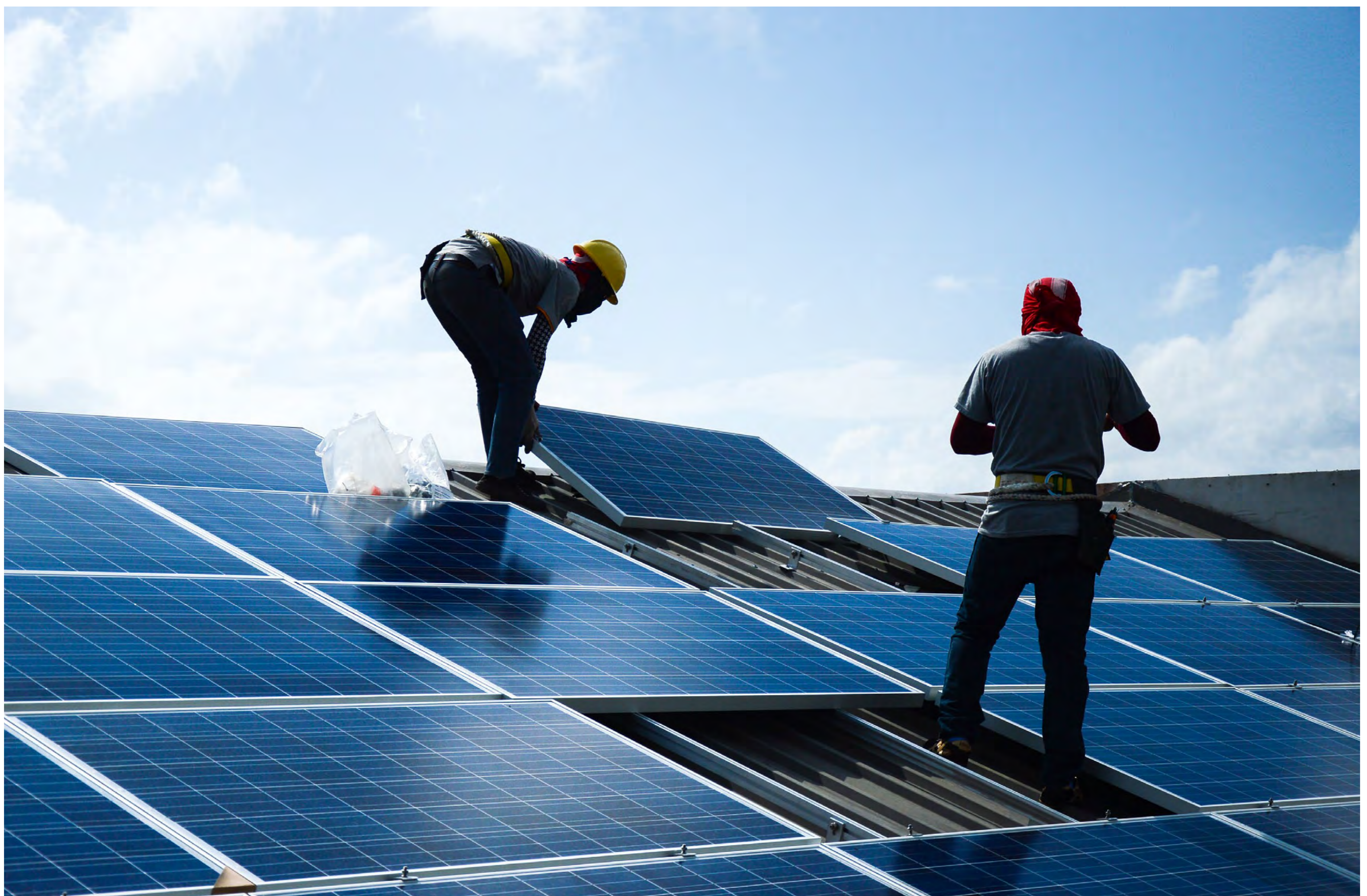
Solar panels will be used on rooftops.
